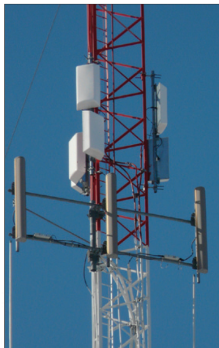
Figure 1: Arcadian Networks' "plug & play" equipment was installed quickly to link 25 Crow Wing substations
