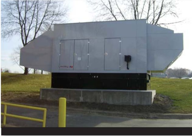
A Connexus distributed-generation installation controlled by 700-MHz wireless communications.
